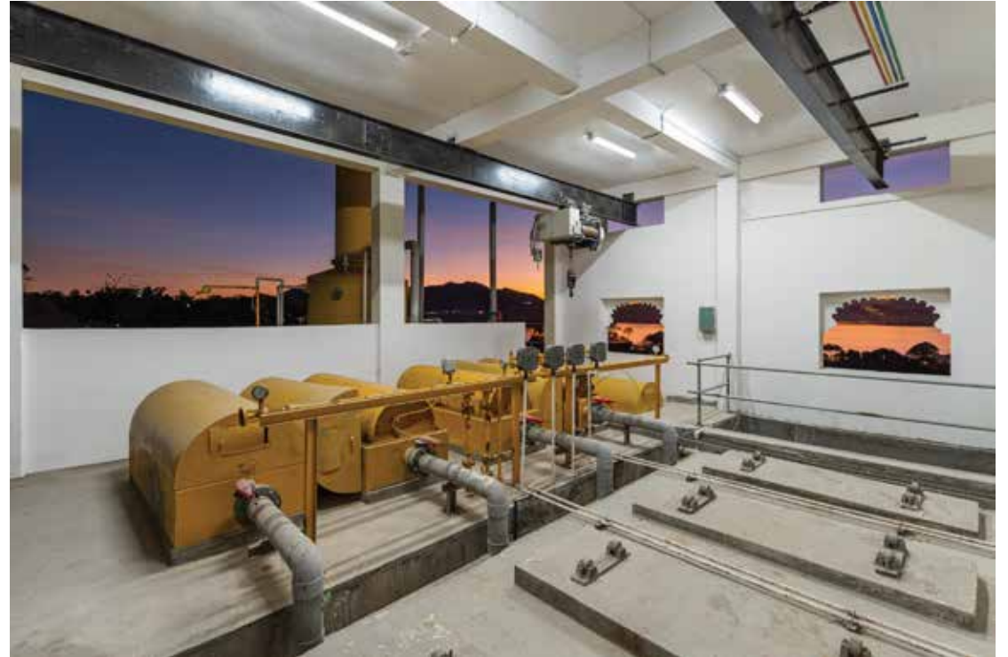
Left : Electric Panel and Control Room Right : Chlorination Chamber
